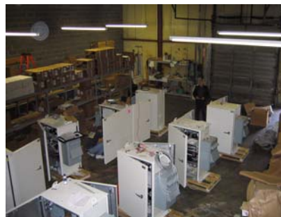
Wiring cabinets before installation
